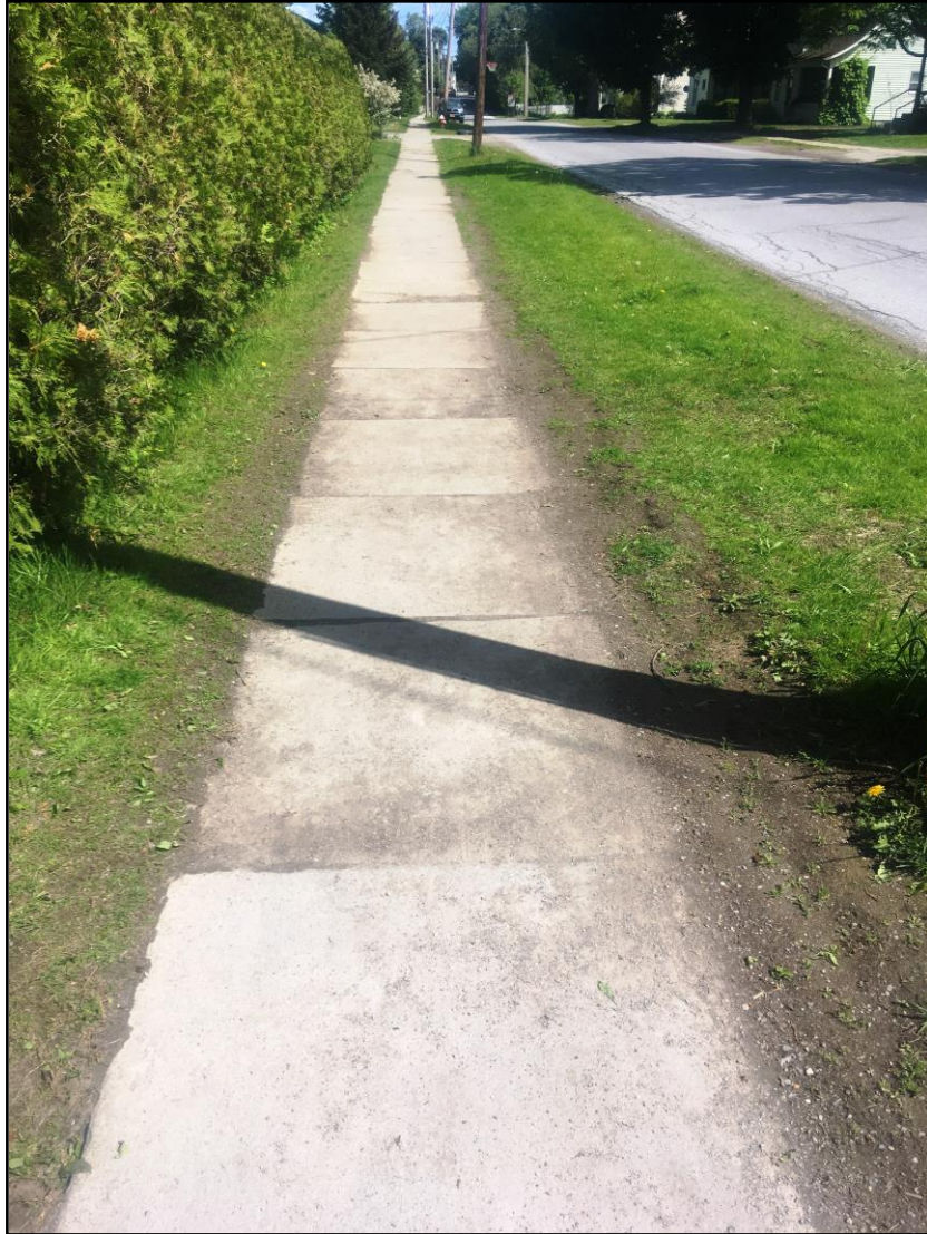
Figure 3. Mountain Street. Sidewalk will need to be elevated to eliminate ponding.
