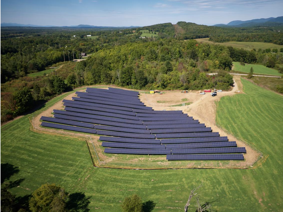
Solar array in Brandon, Vermont constructed by Green Lantern Solar for the Town of Brandon
