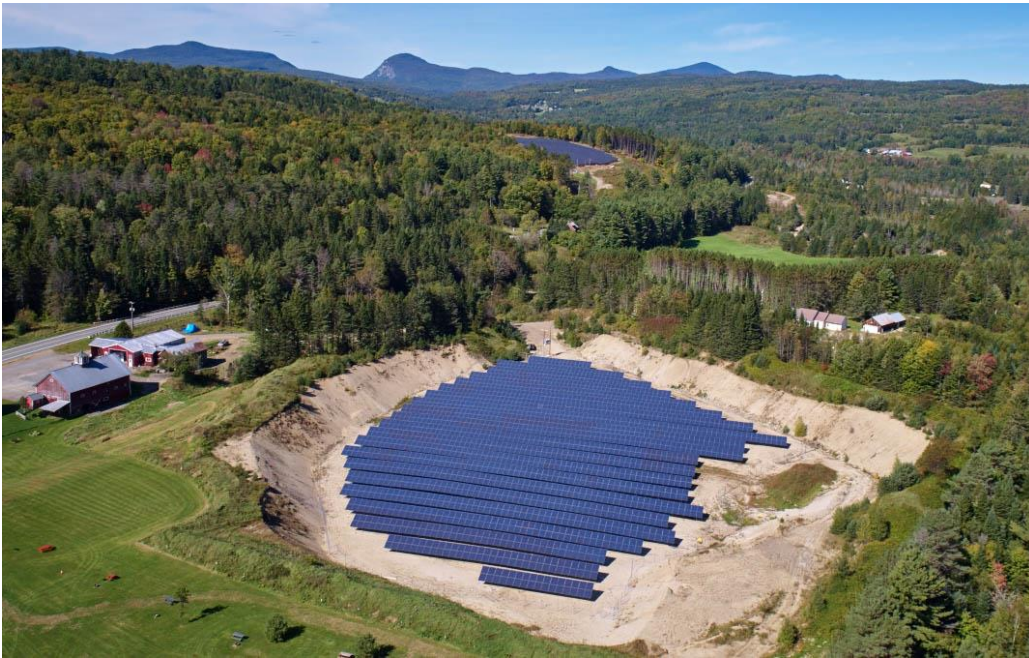
Solar array on a former gravel pit in West Burke, VT constructed by Green Lantern Solar for Lyndon Institute
