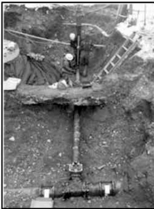
West Street New Hydrant & Valve by the Bank
