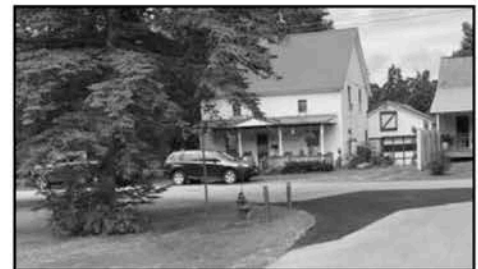
Leak Repair with New Hydrant & Valve on the Corner of Taylor & Elm
