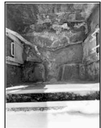
Influent Sewer Structure Clogged with Rags from Items Flushed Daily that Should go in Garbage Can
