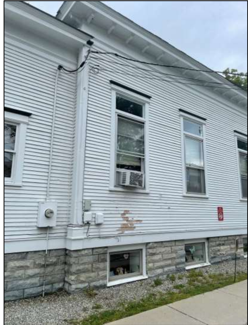
Figure 2. North side peeling paint. (09/10/2021)
