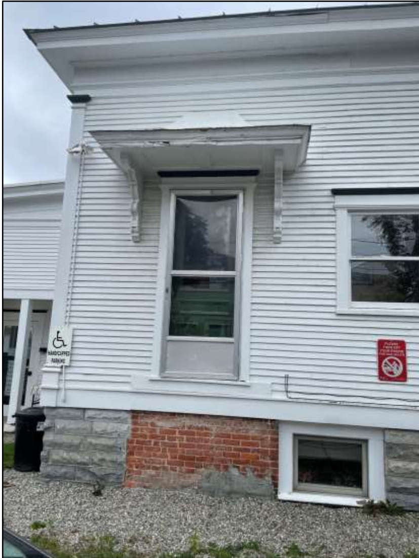
Figure 1. Side door overhang, north side. (09/10/2021)
