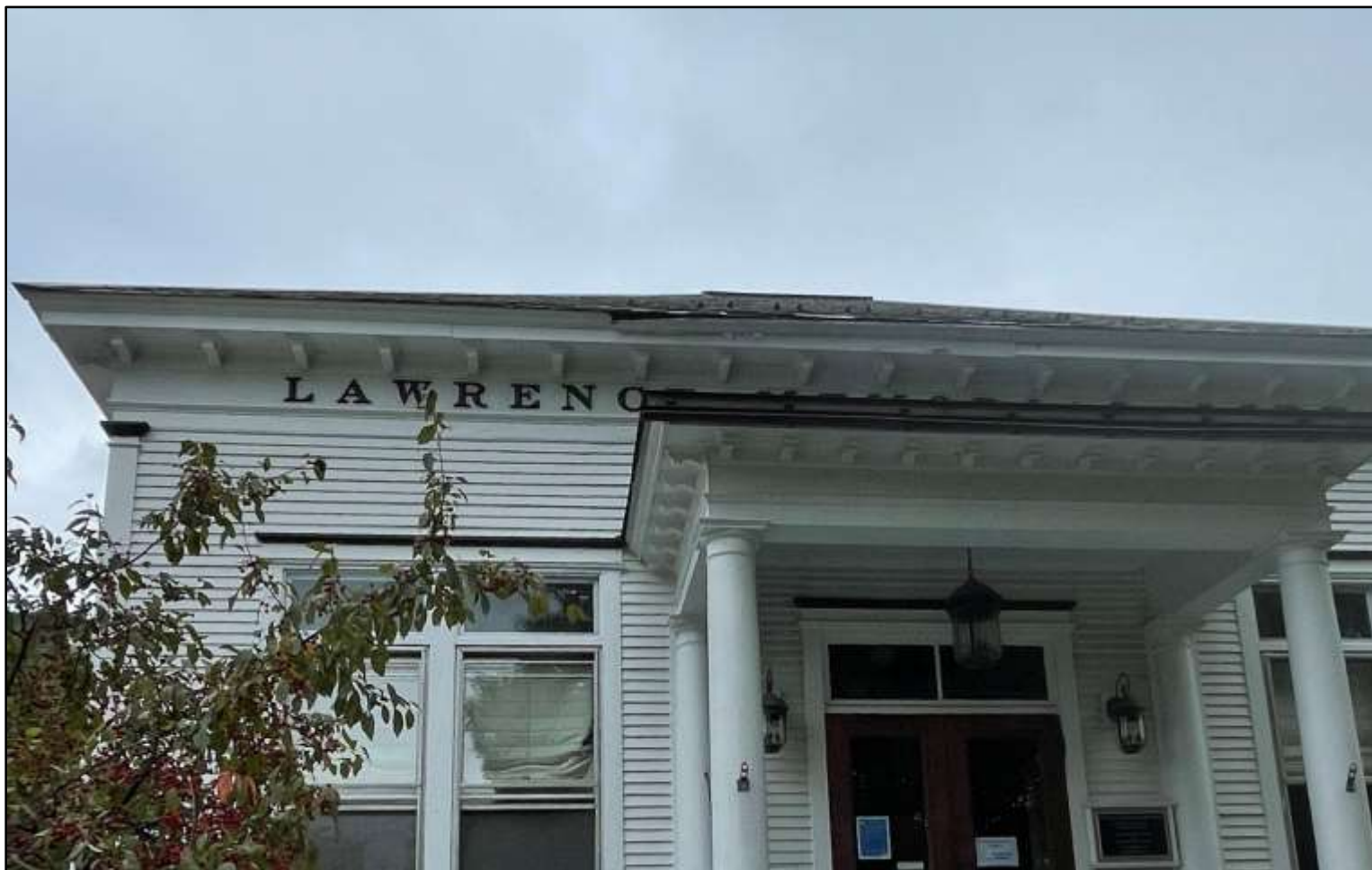
Figure 7. Closer view of upper roof eave deterioration. (09/10/2021)
