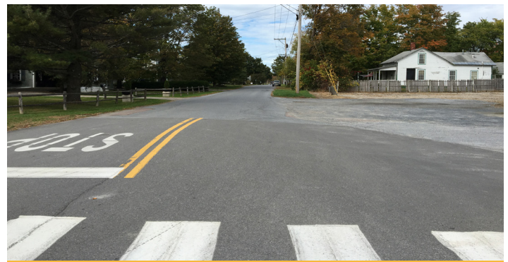
Open access to the Thad’s Automotive & Tire property creates an unsafe area for pedestrians and cyclists.
