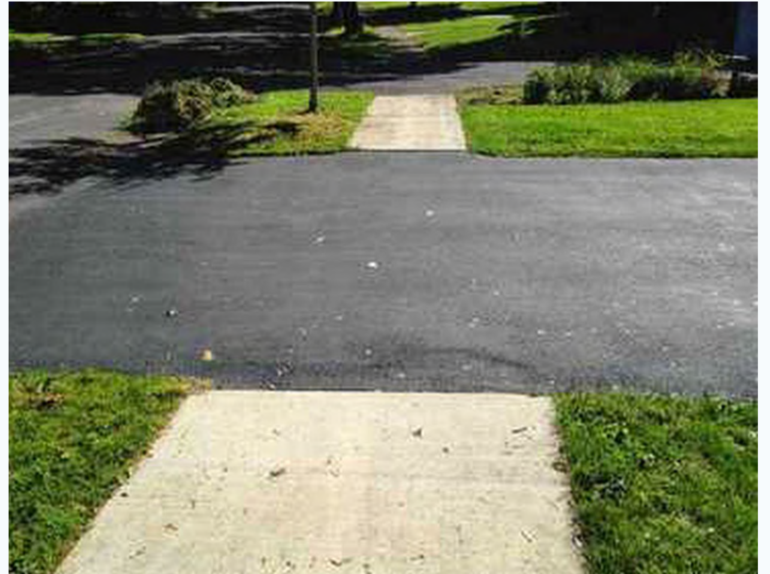
Sidewalk Stops at Driveway
