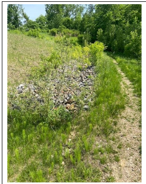
Photo #8 – Stone Drainage Ditch Growth
