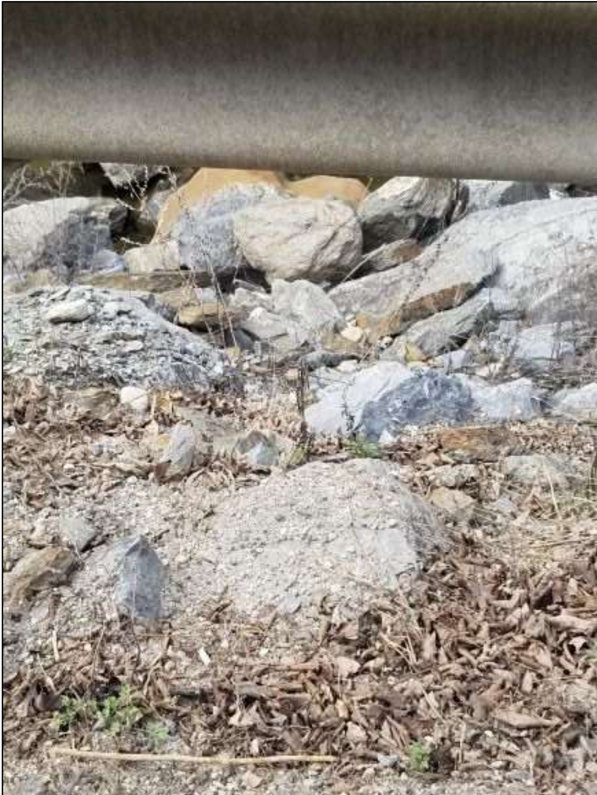
Figure 2. View of the newer slide from the top of the bank and edge of shoulder. (Photo: Cota)
