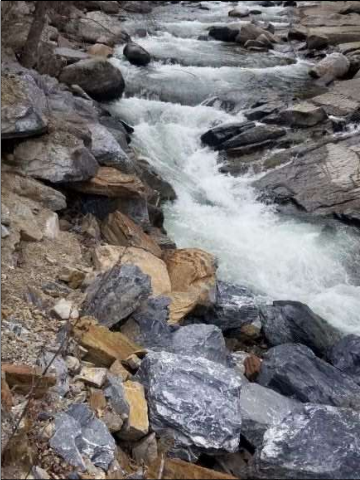
Figure 5. Another view of the older slide with the toe of the slope having being washed away. (Photo: Cota)
