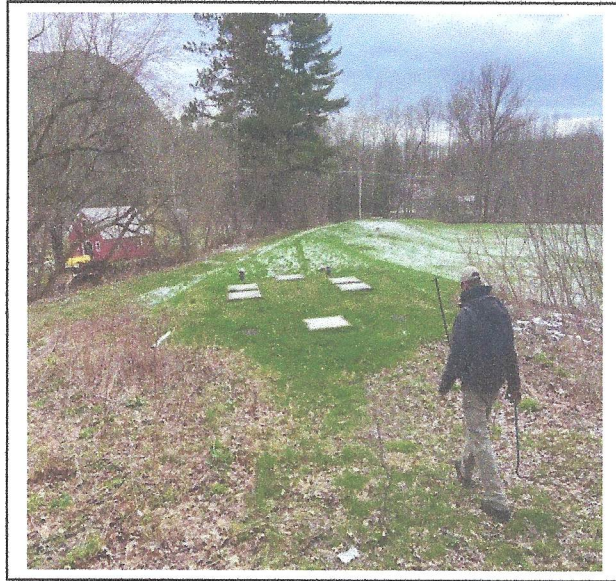
Septic Tank Covers and Disposal Field
