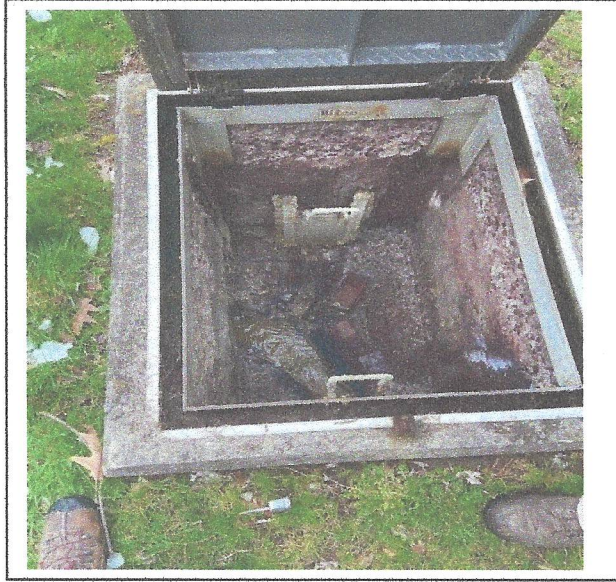
Septic Tank Influent Trough
