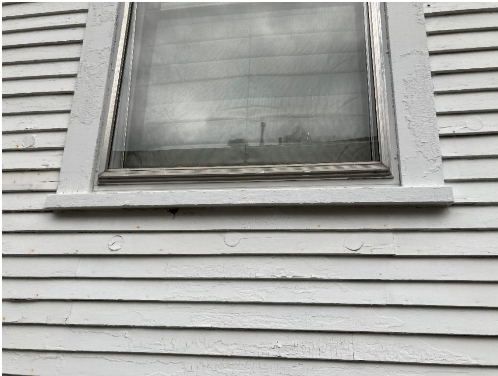
Figure 10 - showing cylindrical holes indicating blown in insulation in the wall cavity from the exterior side.
