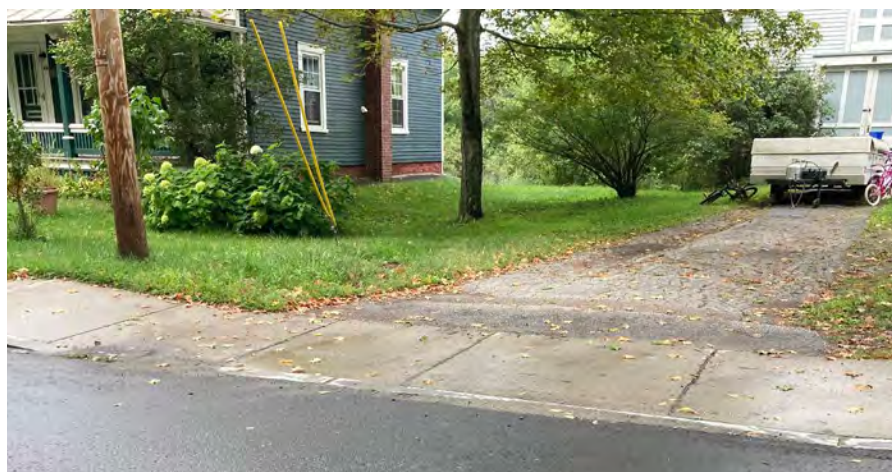
Typical Curbed Sidewalk at Driveway: A continuous concrete sidewalk surface, and curb, dips down to meet the existing driveway grade. See detail at right. While this configuration allows for a continuous surface, the "up and down" sidewalk travel can feel uneven, especially when driveways are close together.
