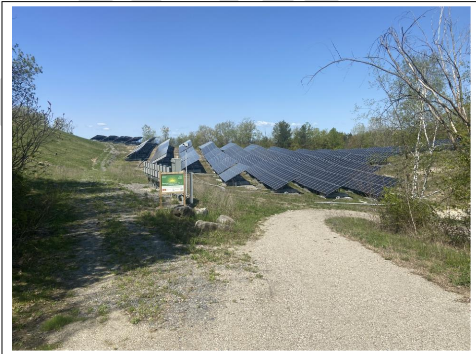
Photo #2 – Solar Array
