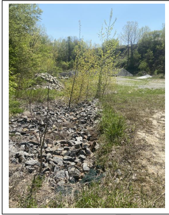
Photo #7 – Stone Drainage Ditch Growth Northeast Corner
