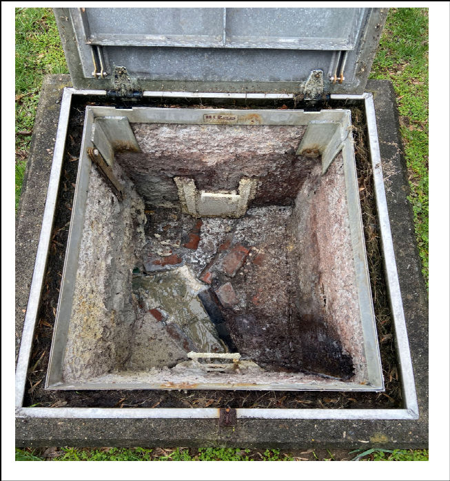
Septic tank outlet trough
