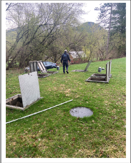
Septic tank access hatches
