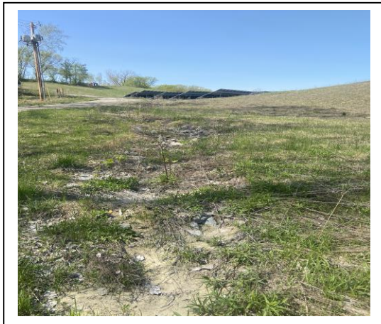
Stormwater Ditch in Need of Reconstruction
