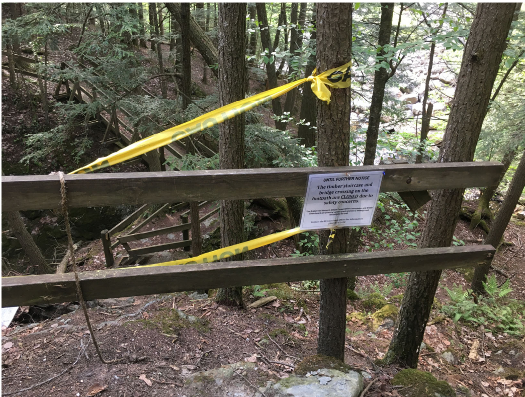
Figure 7. Signage, caution tape, and wooden planking mark the end of the footpath and closure of the bridge crossing at Memorial Park.
