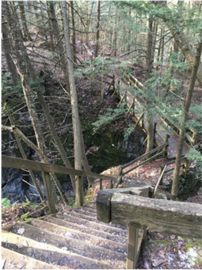
Figure 4. Original wooden staircase leading to footbridge over chasm for viewing Burnham Falls. Due to deteriorating conditions and safety concerns, this staircase was dismantled in the fall of 2019, and the bridge trail was closed until further notice.
