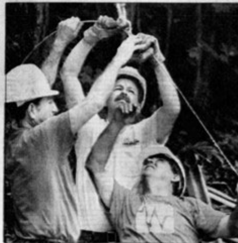
JASON REDMOND, for the Free Press Waitsfield and Champlain Valley Telecom workers set up a line to pull a telephone line out of the New Haven River on Sunday.
