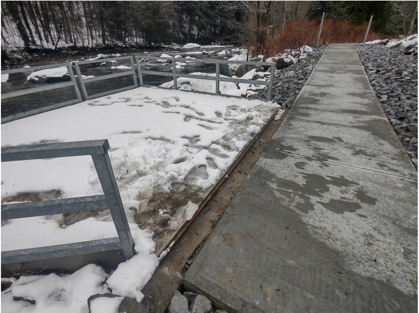
Figure 3: Space between the platform and new walkway where boards were removed at the start of construction.
