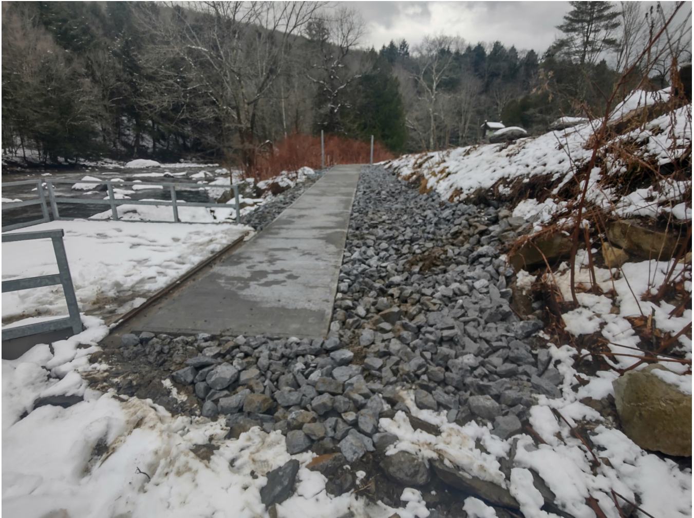
Figure 2: Completed concrete walkway looking downstream. Platform to the left of the photo.
