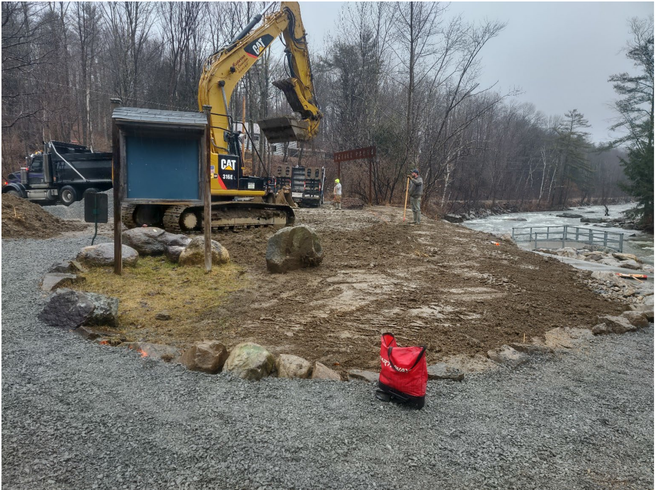
Figure 7: Reshaping of the upper slope and restoration of the lawn area underway. Memorial stone reset to the right of the informational sign in photo. Restored gravel walkway visible in foreground. Split rail fence to be installed in the restored lawn area at edge of parking. Barrier stones to be set as needed once split rail fence has been installed.
