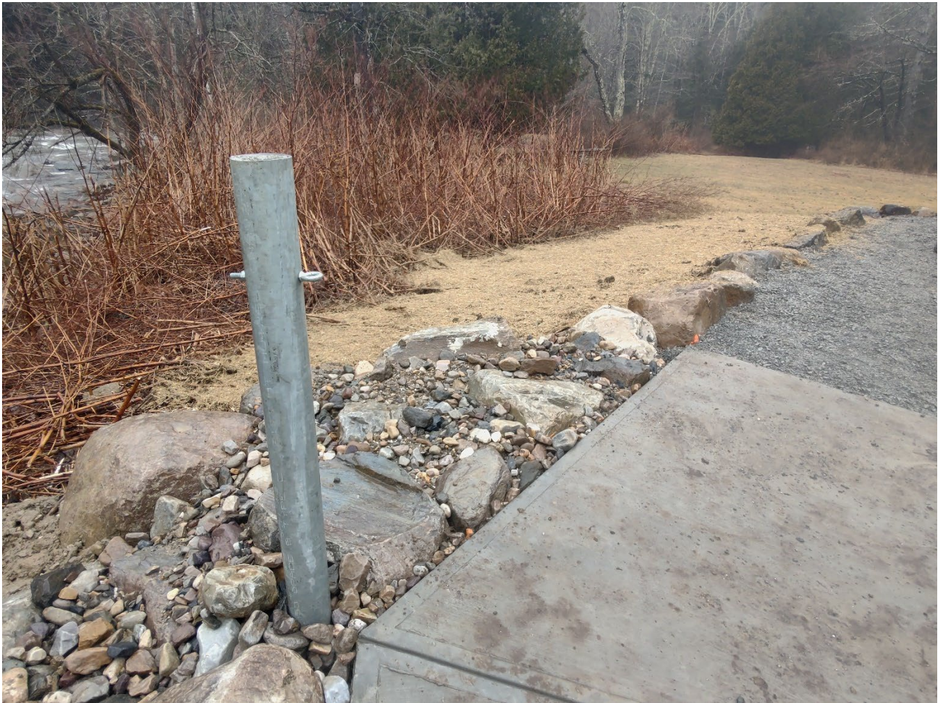
Figure 5: Galvanized post cut to length and filled with concrete. Threaded eye bolt attached to the post. Restored lawn area with seed and mulch visible in background.
