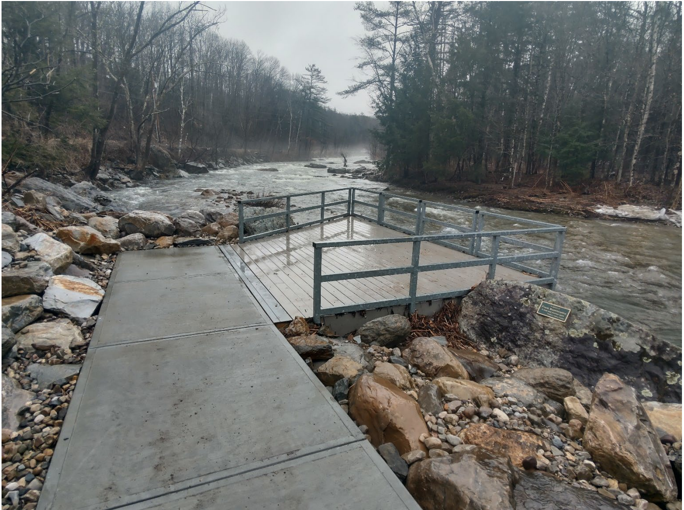
Figure 1: View of newly placed boulders with voids filled with bank run gravel. Note deck boards added to fill gap between platform and concrete walkway.
