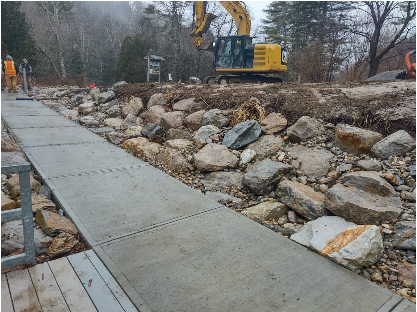
Figure 4: View of completed boulder placement on the parking lot side of the walkway. Work underway to shape top of slope and spread topsoil to restore lawn / planting area.
