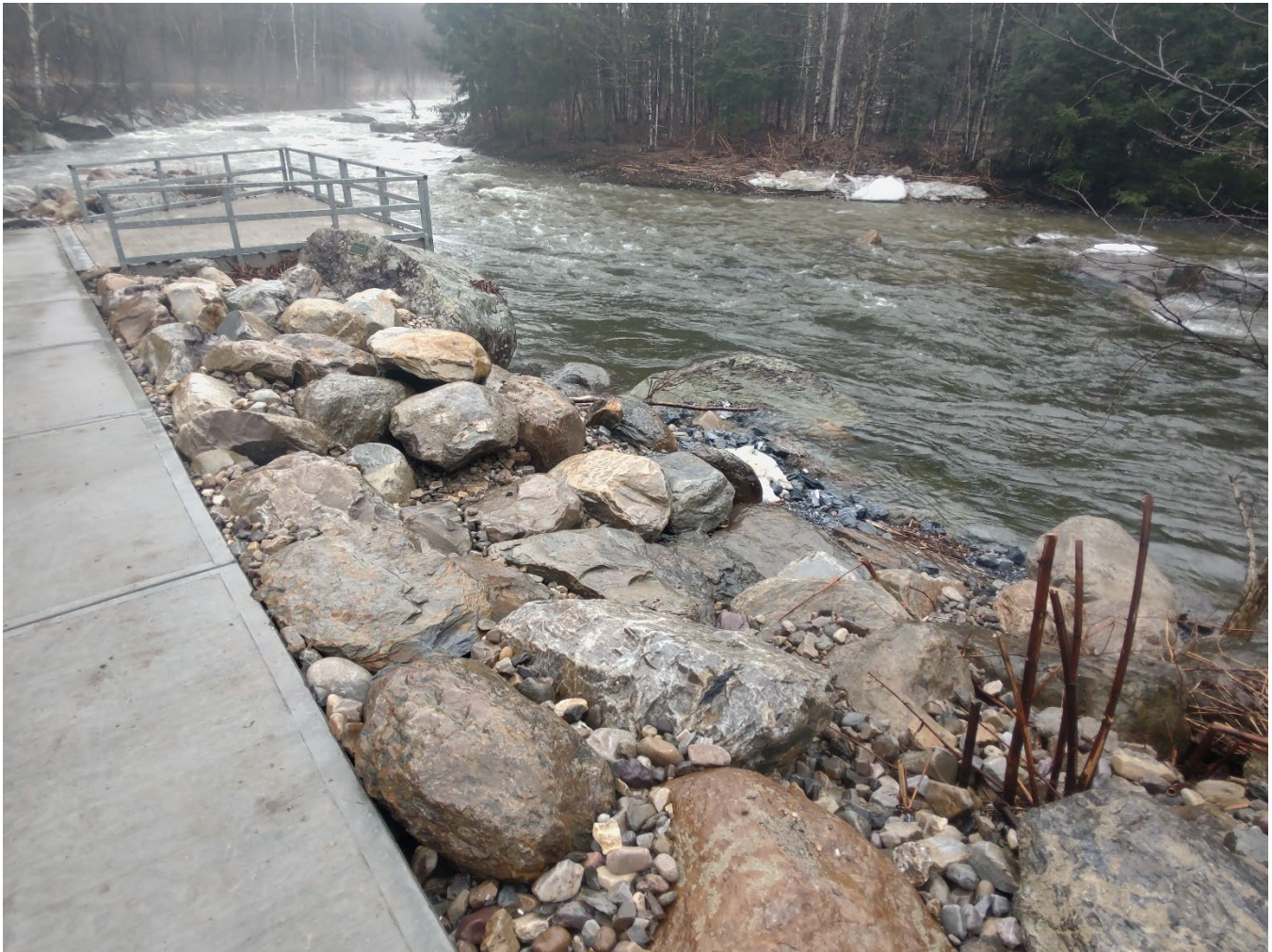
Figure 2: View of completed boulder placement on river side of the walkway with stepping stones placed for access to edge of river.
