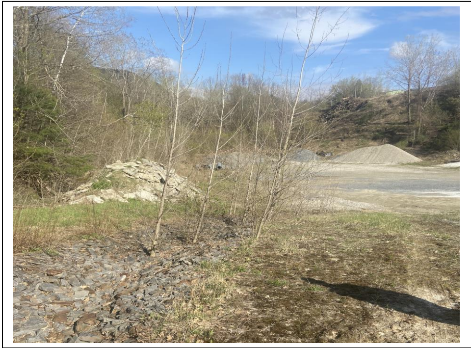
Photo #5 – Drainage Swale In Need of Tree Removal
