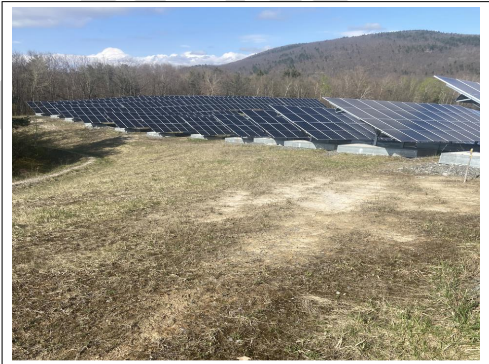
Photo #2 – Area in Need of Vegetative Cover
