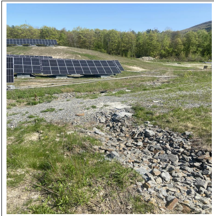
Photo #8 – Filled Stone Drainage Ditch In Need of Culvert
