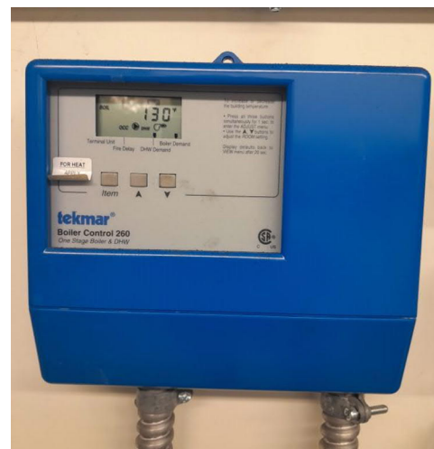
Figure 43 – Existing Boiler Controller
