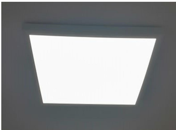
Figure 56 – Existing LED Panel Fixture
