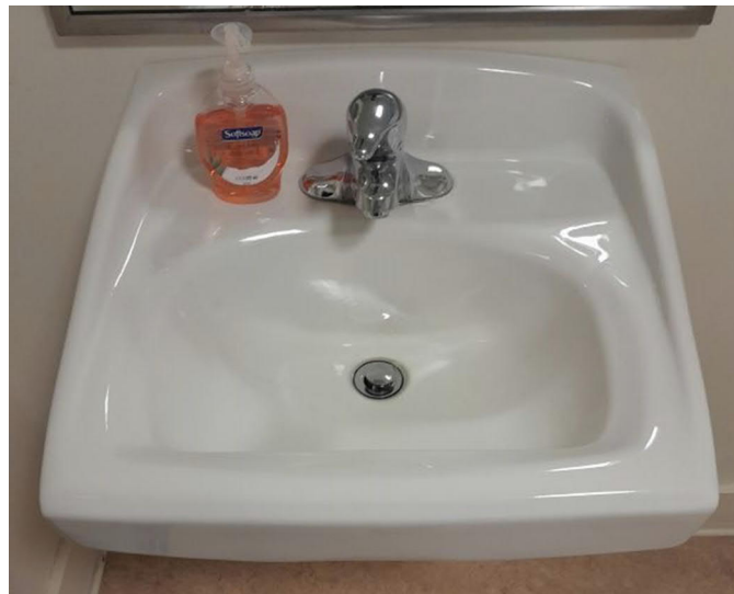
Figure 58 – Existing Lavatory Faucet
