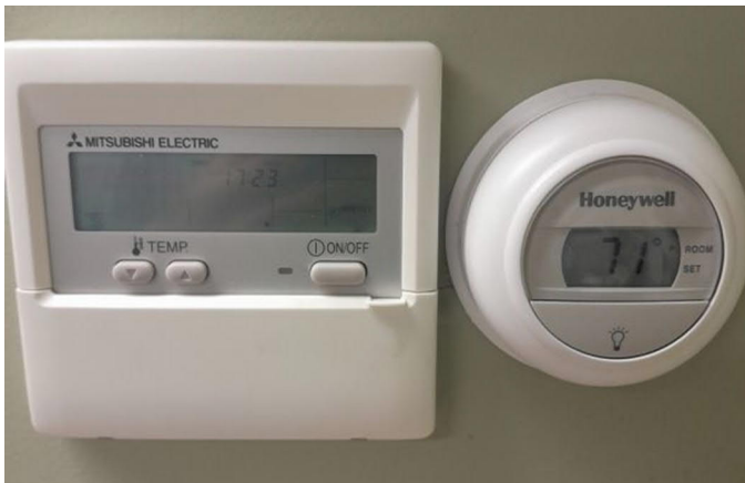
Figure 50 – Existing Programmable Thermostats
