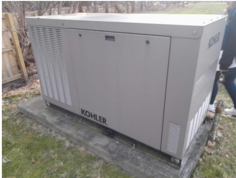
Figure 3 – Existing Propane-Fired Generator
