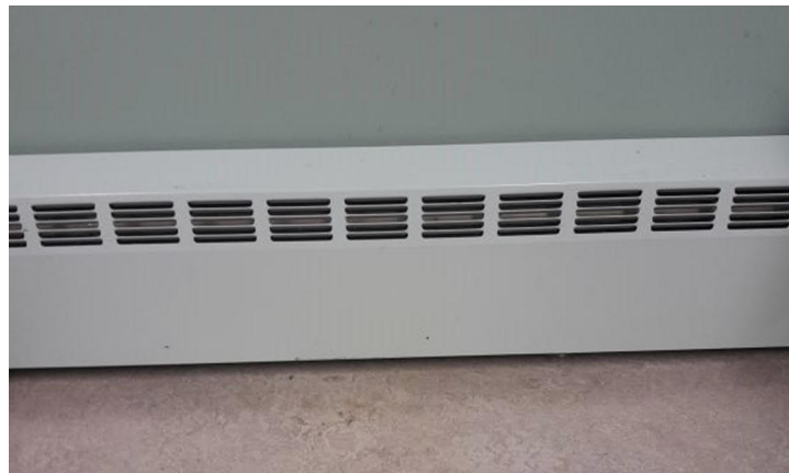
Figure 51 – Existing Fin-Tube Radiator
