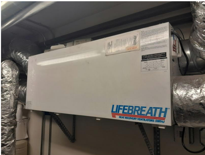
Figure 46 – Existing Heat Recovery Ventilator
