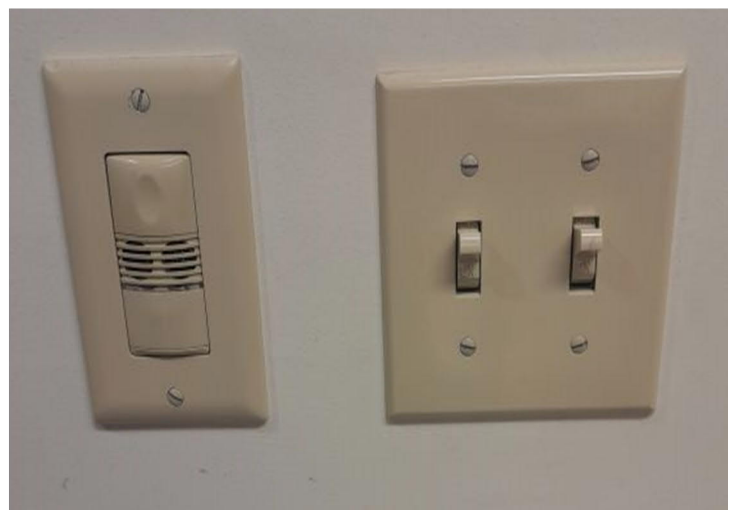
Figure 55 – Existing Wall Mounted Light Switches
