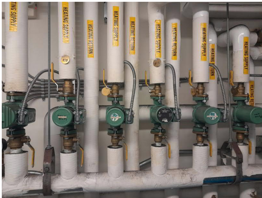
Figure 45 – Existing Hot Water Circulation Pumps
