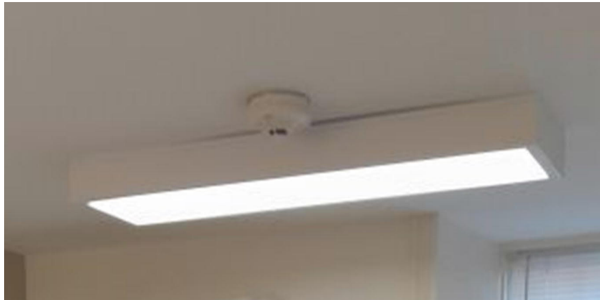
Figure 57 – Existing Ceiling Mounted LED's
