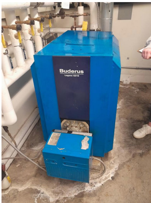
Figure 44 – Existing Oil-Fired Boiler
