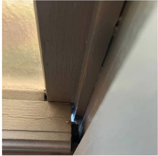
Figure 30 - Air leakage at the meeting rail.
