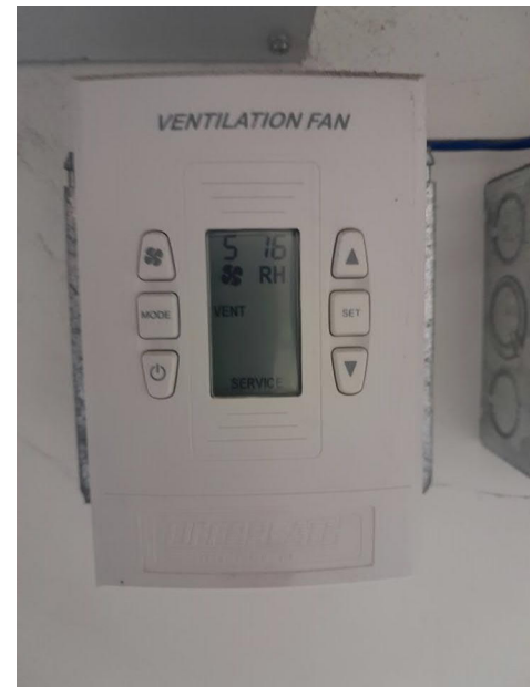
Figure 47 – Existing Ventilation Fan Controller
