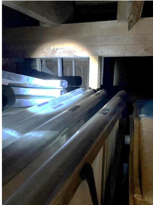
Figure 22 – Looking at the back wall under the stage we could see the open framed wall with no insulation.
