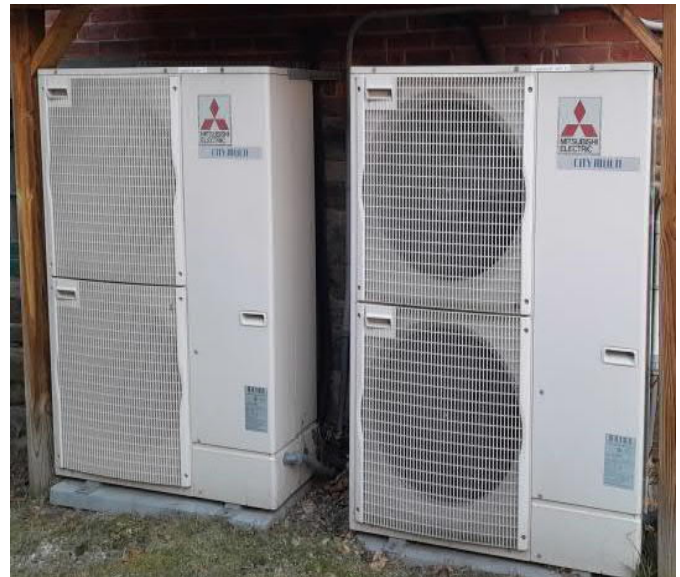
Figure 49 – Existing Exterior Heat Pump Units
