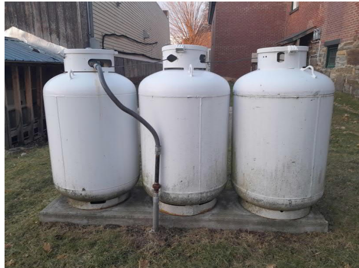
Figure 1 – Existing Propane Storage Tanks
