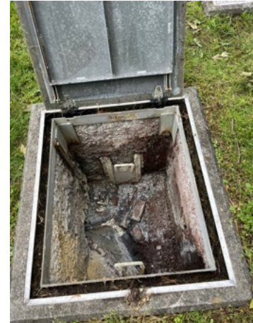
Deteriorating effluent sewer structure before rehabilitation
