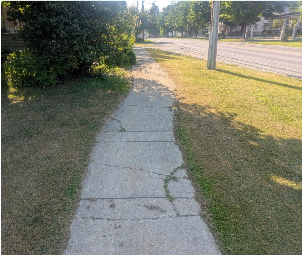
Photo 2 Deteriorated Concrete and Substandard (Four-Foot) Width
