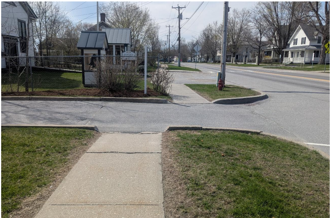
Photo 5 Misaligned Sidewalk Jogs
