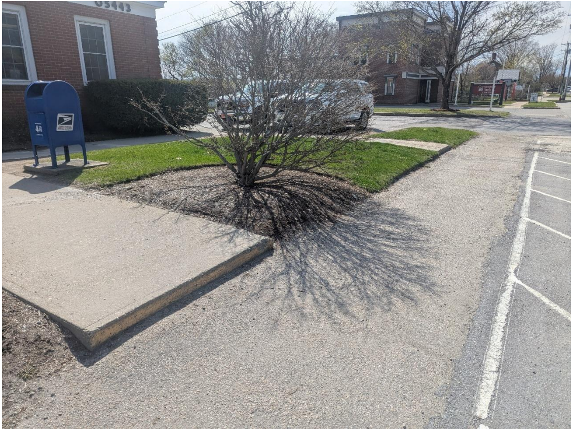
Photo 4 Inaccessible Grade Separation
